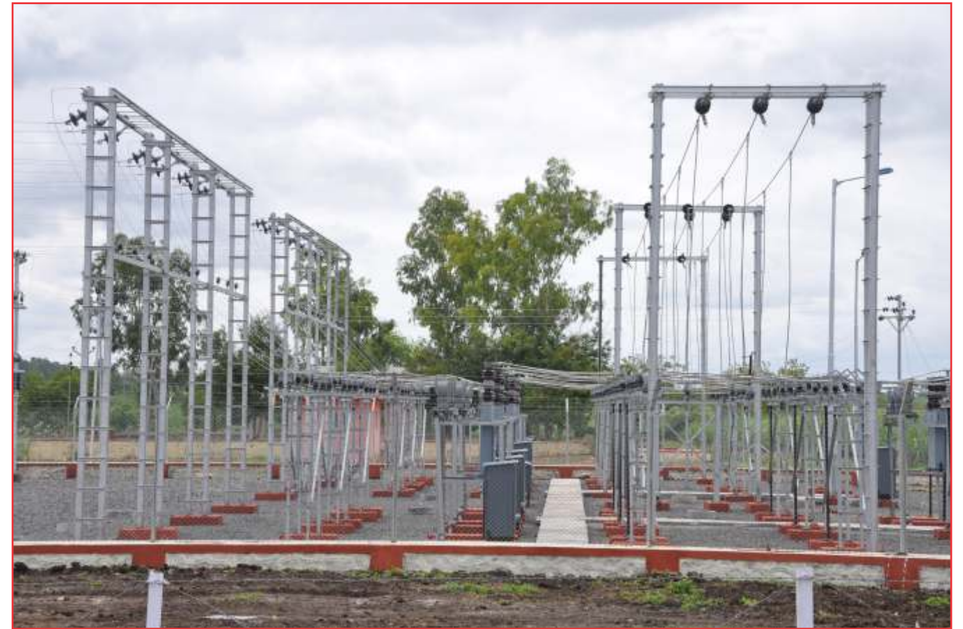
33/11 KV Substation Sansar, Indapur, District Pune
