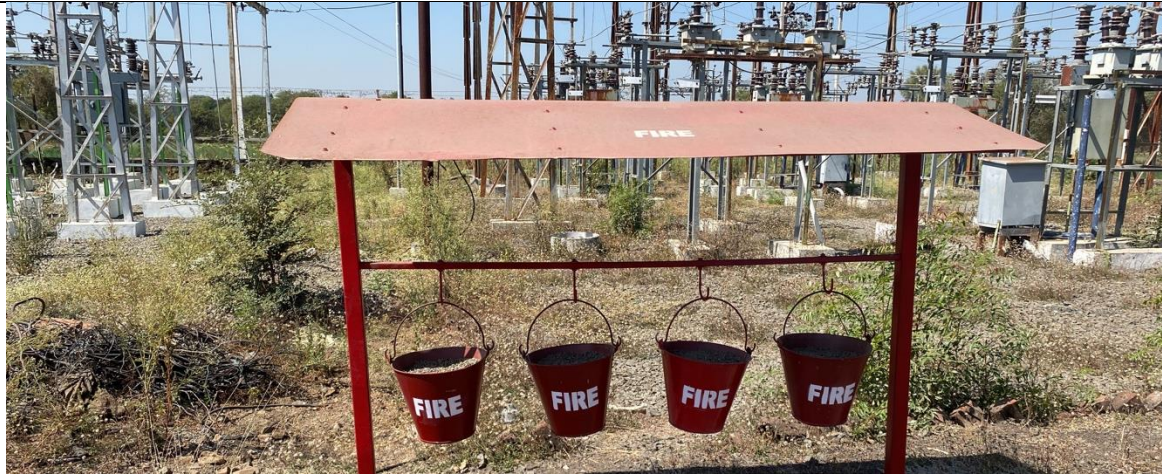
Fire buckets at substation
