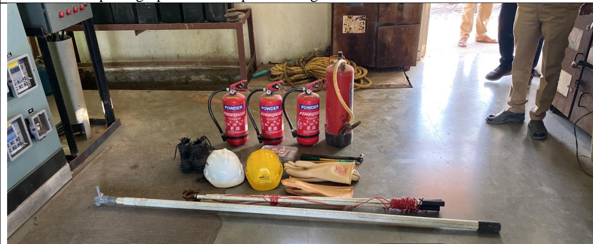
Safety equipments at substation
