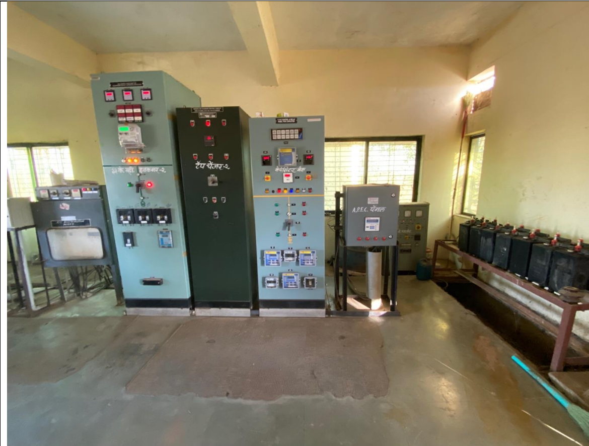
Control room photograph of Bhadarpur existing substation
