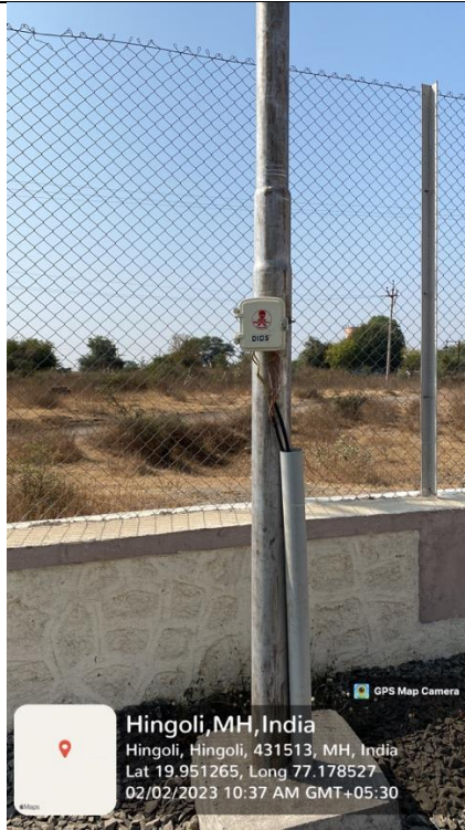
Safety sign at the pole
