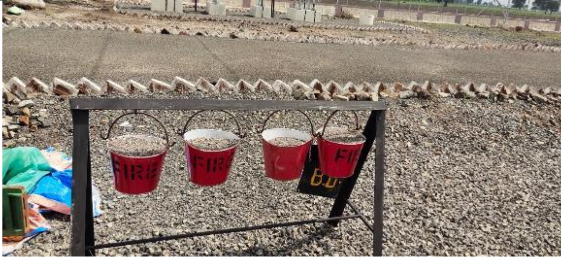
Firefighting sand buckets at substation
