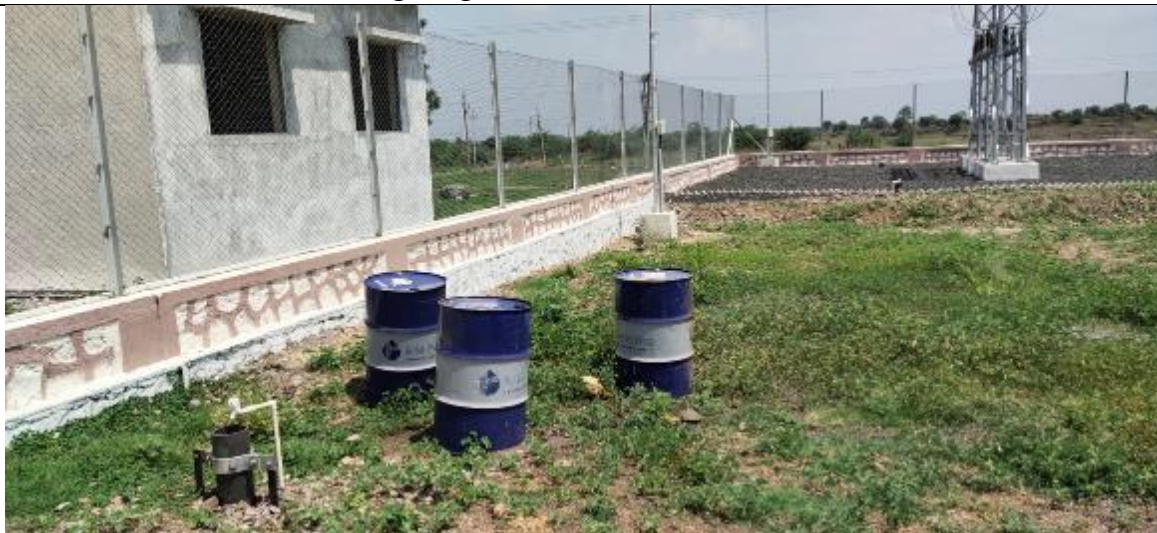
Transformer oil drums kept within substation premises
