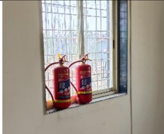
Fire extinguishers at substations
