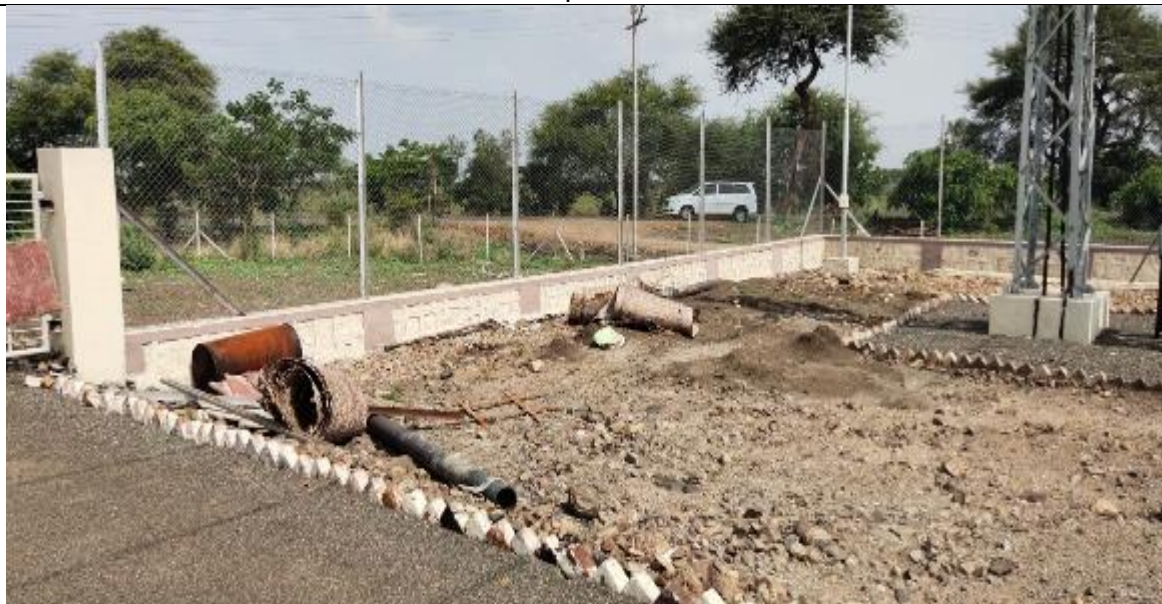
Scrap waste within substation
