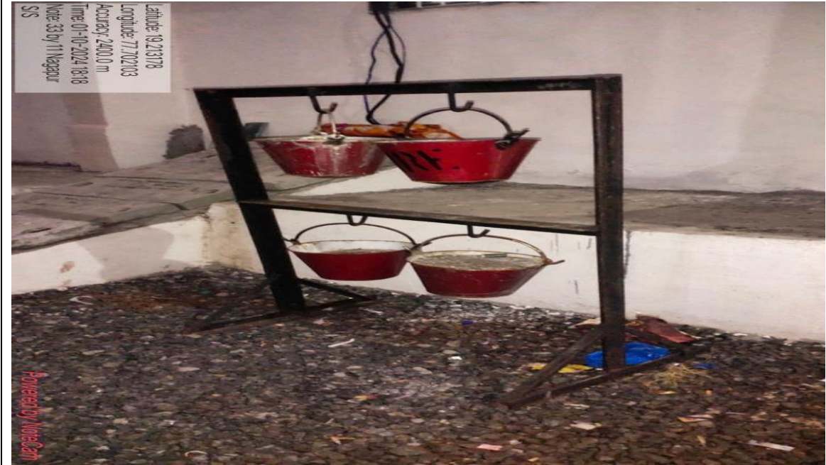
Fire buckets at substation
