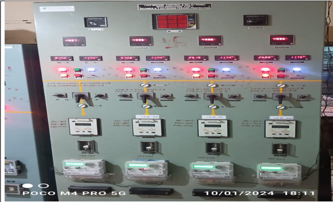
Control room Photograph for Pardi Substation
