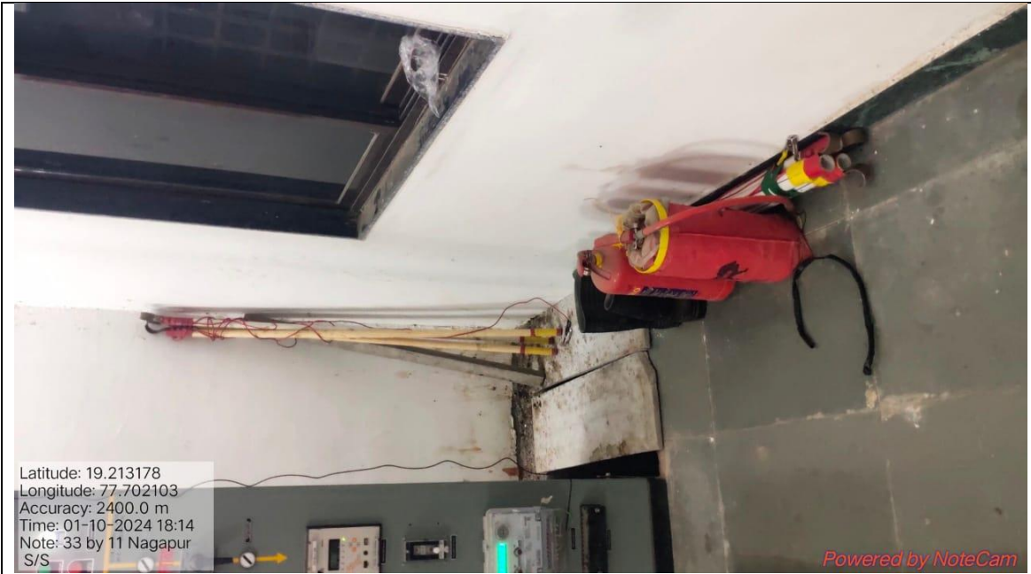
Safety Equipment in Substations
